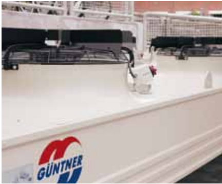
top: Green cooling with a transcritical carbon dioxide refrigeration system
