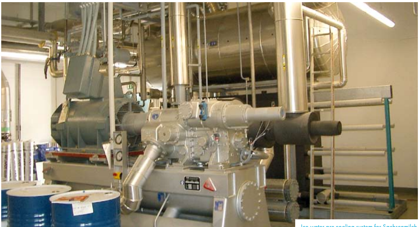
Ice water pre-cooling system for Sachsenmilch
