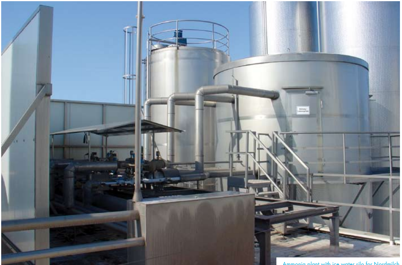
Ammonia plant with ice water silo for Nordmilch
