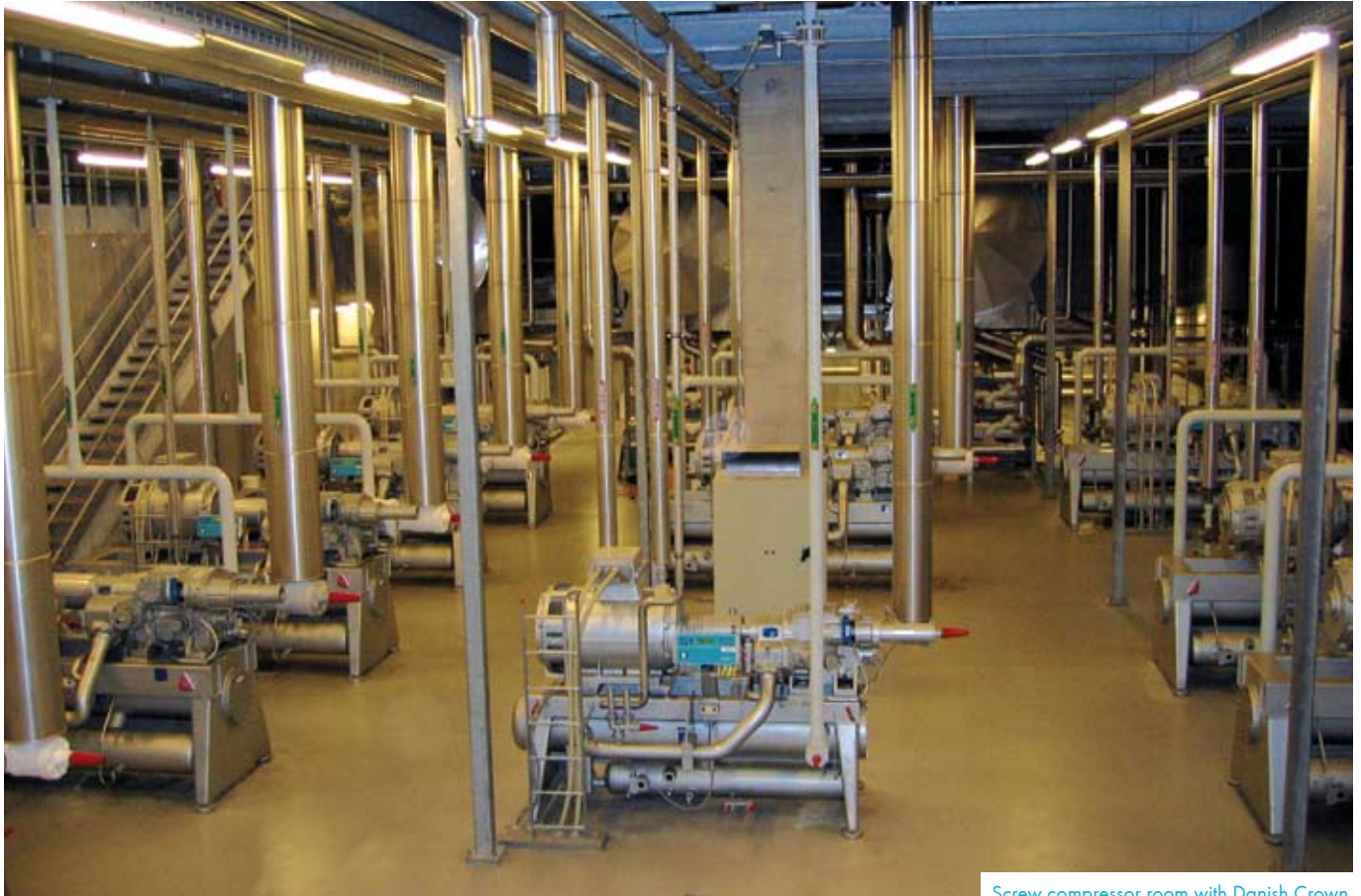
Screw compressor room with Danish Crown
