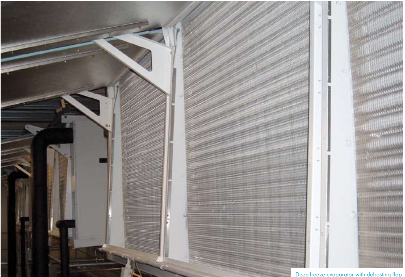
Deep-freeze evaporator with defrosting flap
