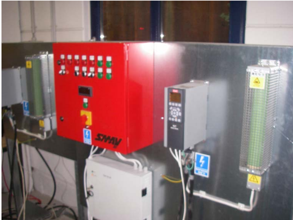
Fig. 1 Control unit, power supply and frequency converter for supply air and outlet air unit
