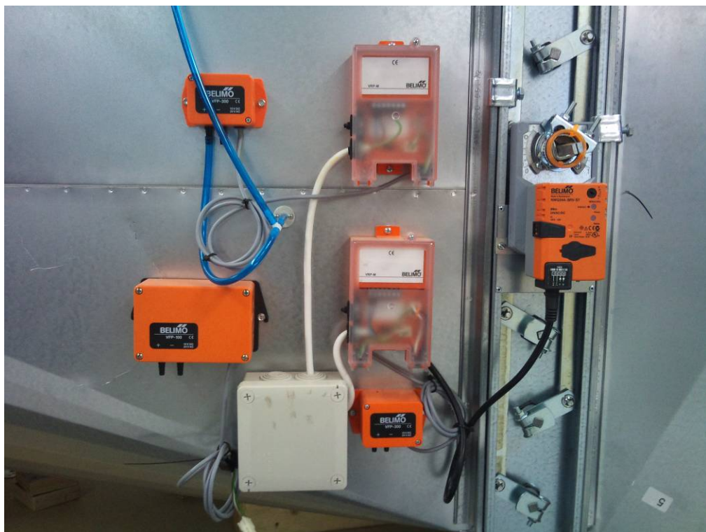
Fig. 5 SAFETY WAY® control components of supply air unit with louver damper SMAY PWII-S
