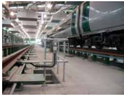
Laois Train Depot in Portlaoise, Ireland 21 CO, 5 CH 4 -Detectors
